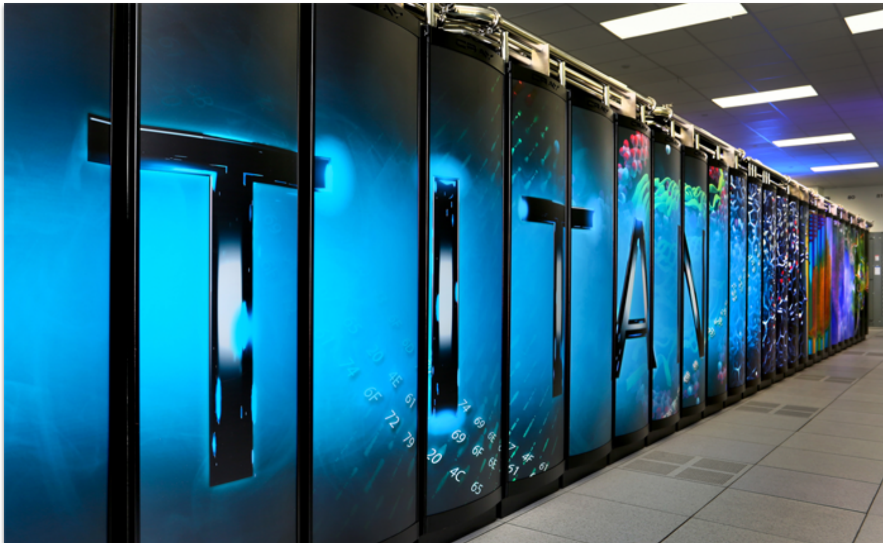
OakRidge Titan Supercomputer (Cray low-latency interconnect)
